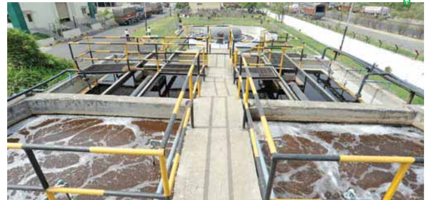
The Effluent Treatment Plant at Dabur's Pantnagar unit
